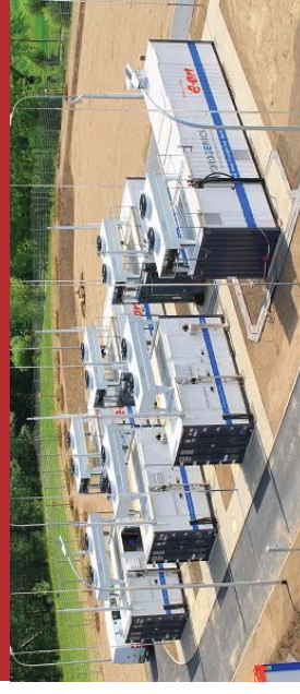
FIGURE 83: E.ON INNOVATION CENTRE ENERGY STORAGE 'POWER TO GAS' PROJECT, FALKENHAGEN, GERMANY SOURCE: HYDROGENICS
