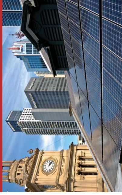
FIGURE 54: SOLAR PHOTOVOLTAIC ROOF SYDNEY TOWN HALL SOURCE: CITY OF SYDNEY
