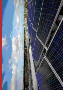
FIGURE 7: SOLAR PV, SURRY HILLS LIBRARY
