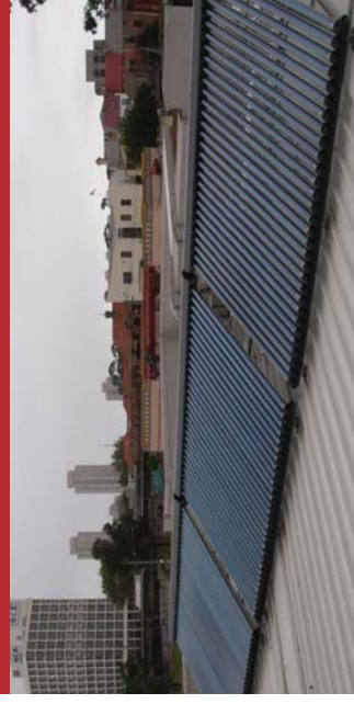
FIGURE 56: SOLAR THERMAL HOT WATER, REDFERN COMMUNITY CENTRE, SYDNEY SOURCE: CITY OF SYDNEY
